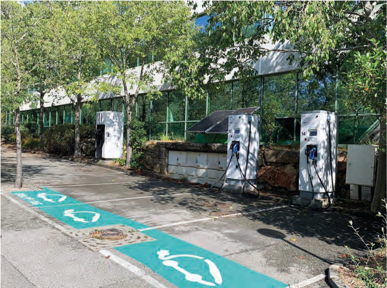
Charging stations at SAP in Mougins
