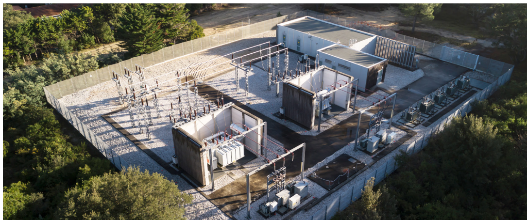
Figure 3: a primary substation [63 kV to 20 kV] in Cap Ferret
