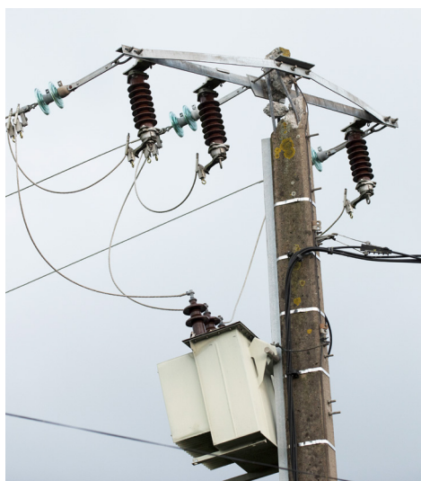
Figure 4: overhead public distribution substation: MV network on the left, MV/LV transformer on a pole, twisted LV network on the right.
